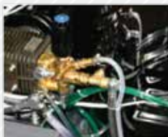
Pressure regulator and safety valve
