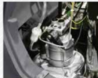
Aluminium boiler ventilator and fuel pump
